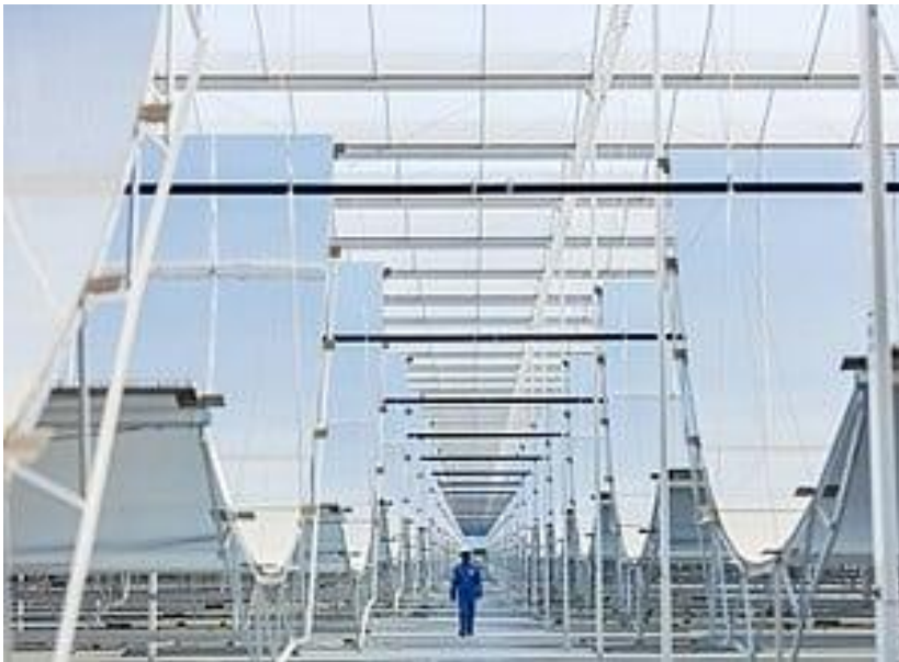
Image 1: AS-Schneider valves are being successfully used at the Amal oilfield in Oman which uses steam generated at the Miraah solar thermal facility.
